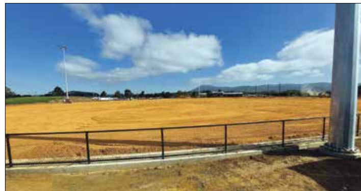
The foundation for the new football oval at the New Gisborne sporting complex has been laid.
